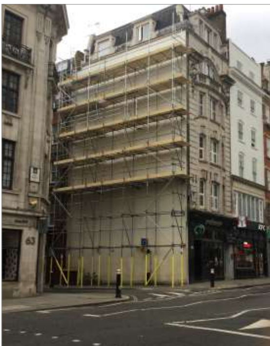
Fig. 3. The scaffolding at the end of August 2021: the wall is ready for the border and hour lines to be painted.
